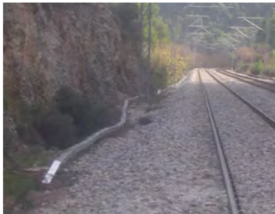
Electrification pole and cable channels in the cess drains, hindering the water flow (drainage). Danger of pounded water.
