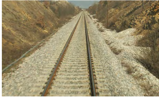
Cess drain plugged by old ballast.
