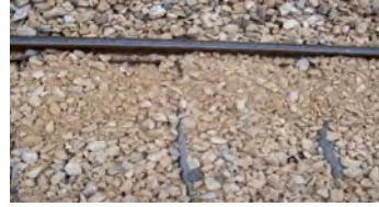
Unsuitable ballast in track
