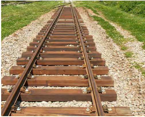
Renovation of a track in a railway station. The track is laid in a "vessel". Water cannot be drained.
