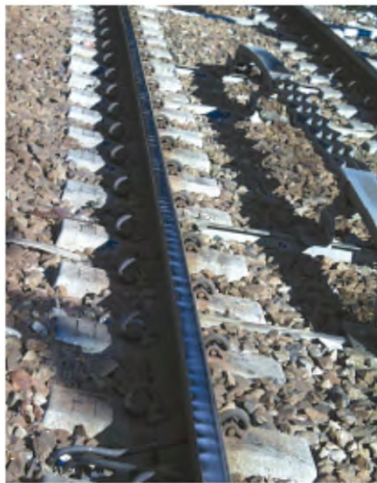
Corrugation - Short wave length track irregularity
