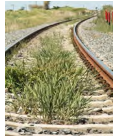
Vegetation in a track with unsuitable ballast
